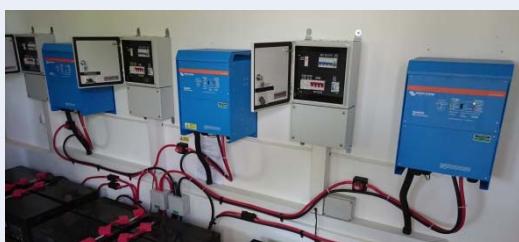
The bespoke Wattstor energy management and storage system
