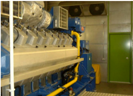
Internal combustion engine CHP plant
