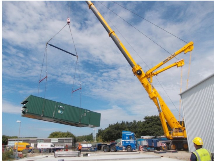
Edina CHP Container offloaded at Crossness STW
